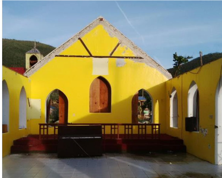
Demolished church in Great Harbor on Jost Van Dyke, awaiting a new roof. The pews and altar had been moved to an adjacent tent.
